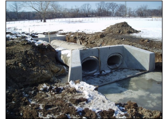
Two pipes allow the swale to go under a farm road
