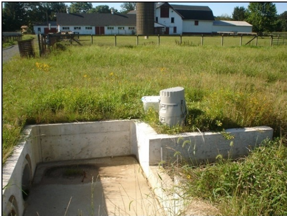
Monitoring equipment at the inlet of the swale
