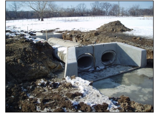
Two pipes allow the swale to go under a farm road
